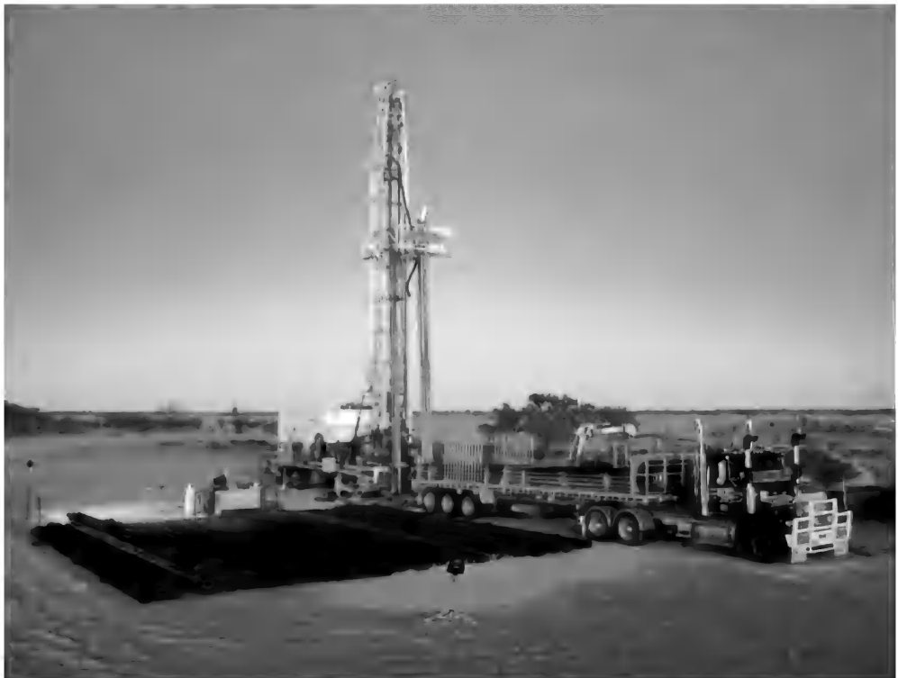
Figure 6. A rotary drill rig being used on a 1200-metre bore in the Great Artesian Basin (Source: Daly Brothers Drilling; available at http://www.dalybros.com.au/ ).
